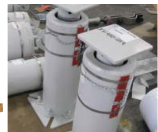
CHAINED TRAVEL STOPS ON VARIABLE SPRING SUPPORTS
